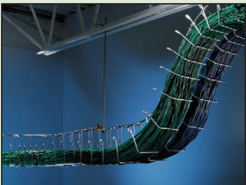
201D Series Snake Tray for Overhead, Under Floors and on Walls
